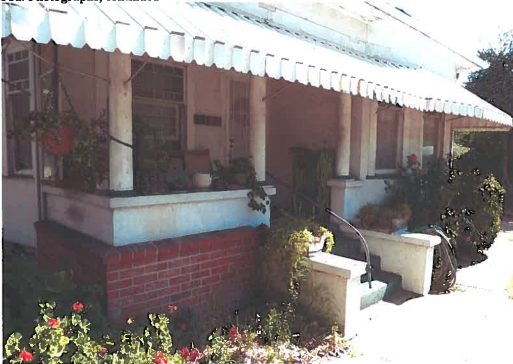
Detail of porch and main entrance at primary (south) façade, July 16, 2010 (Architectural Resources Group)
