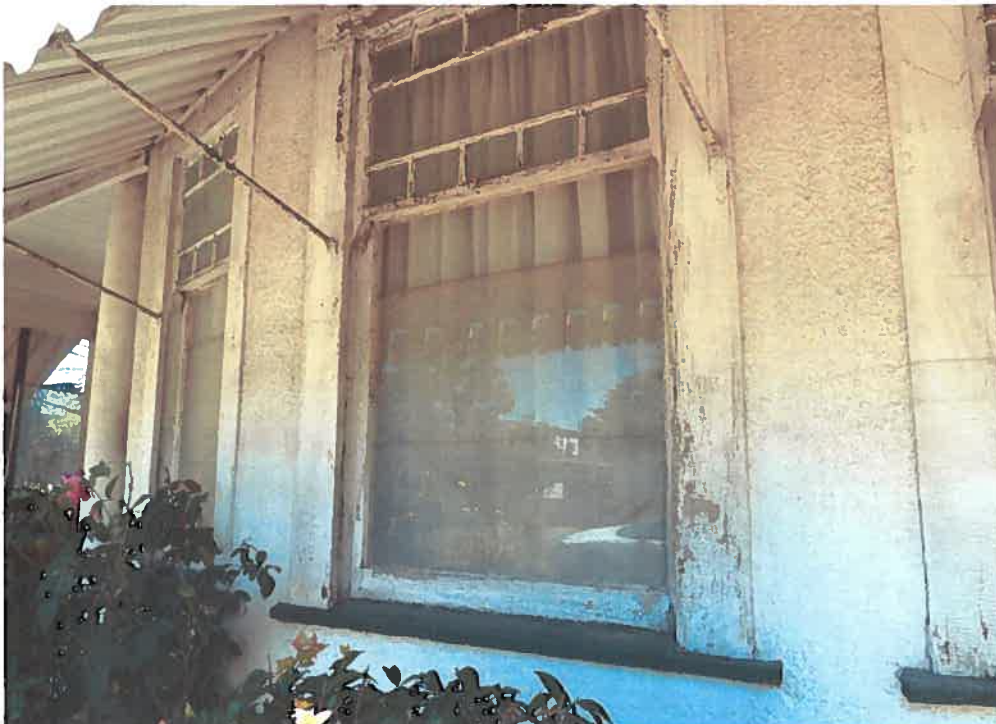
Detail of bay window at primary (south) façade, July 16, 2010 (Architectural Resources Group)
