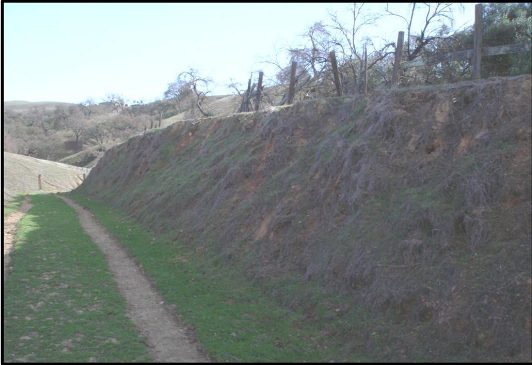
Figure 6: Cut Slope which Exceeds a 25-Percent Grade.
