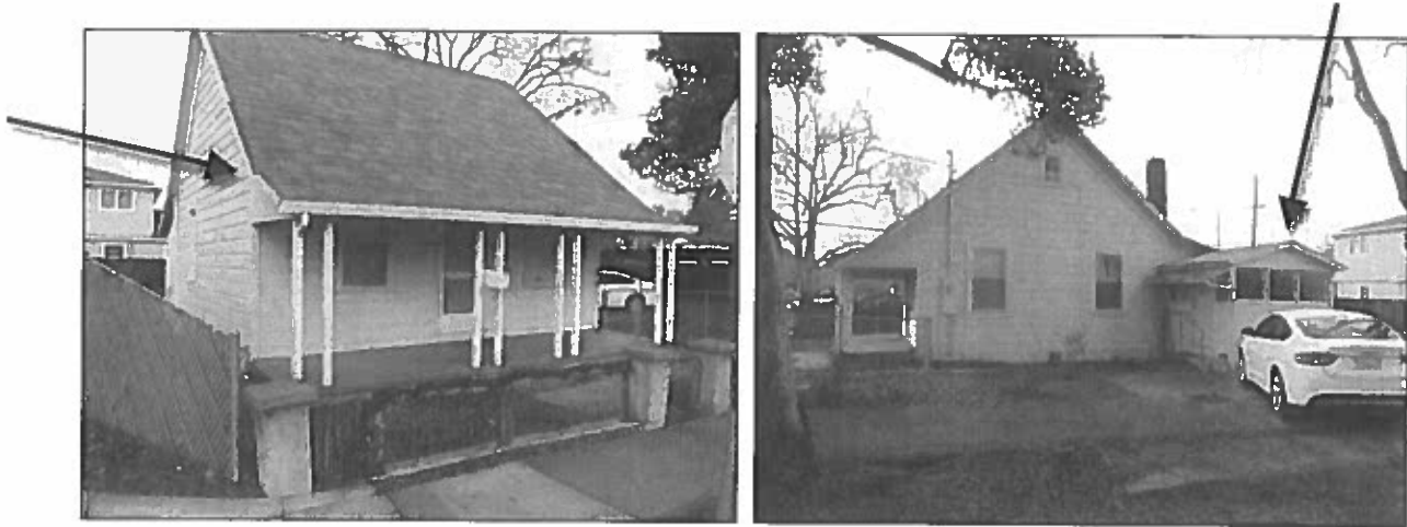
Figures 6 and 7. Left image shows the full width, front porch addition. Note the change in roof pitch that indicates where the porch's shed roof was connected to the main house roof (arrow). Right image shows the right side elevation, with an addition to the right side elevation shown with an arrow.
