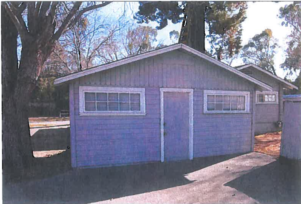
View of front façade of storage building. Laundry room at rear of small residence is visible at right. View to east
