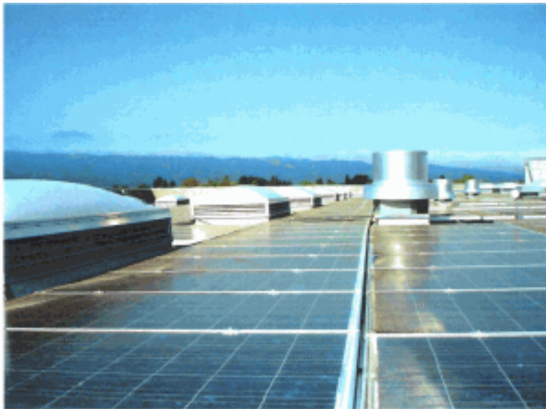
Solar panels on the roof of Borg Fencing Company
