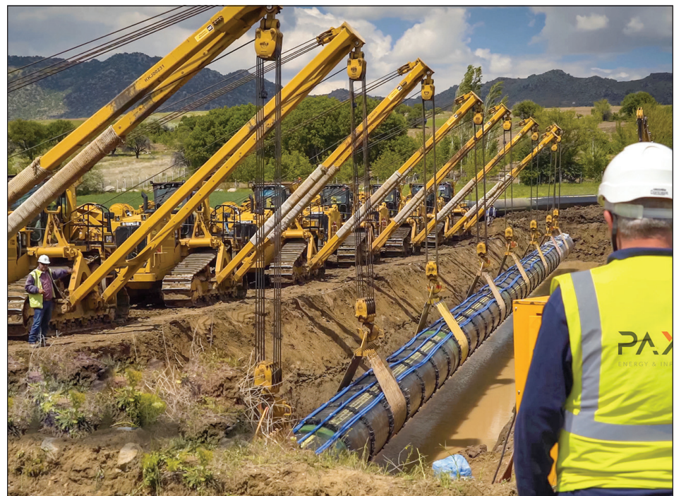
Paxon is a leader in addressing the extensive upgrades required for our nation's electric grid, and local gas systems.
