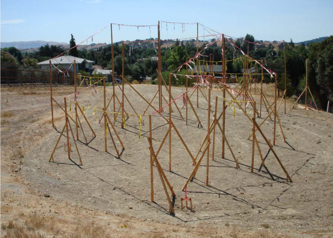
Figure 10: Close-up of the story pole installation from the northwest corner of the site.
