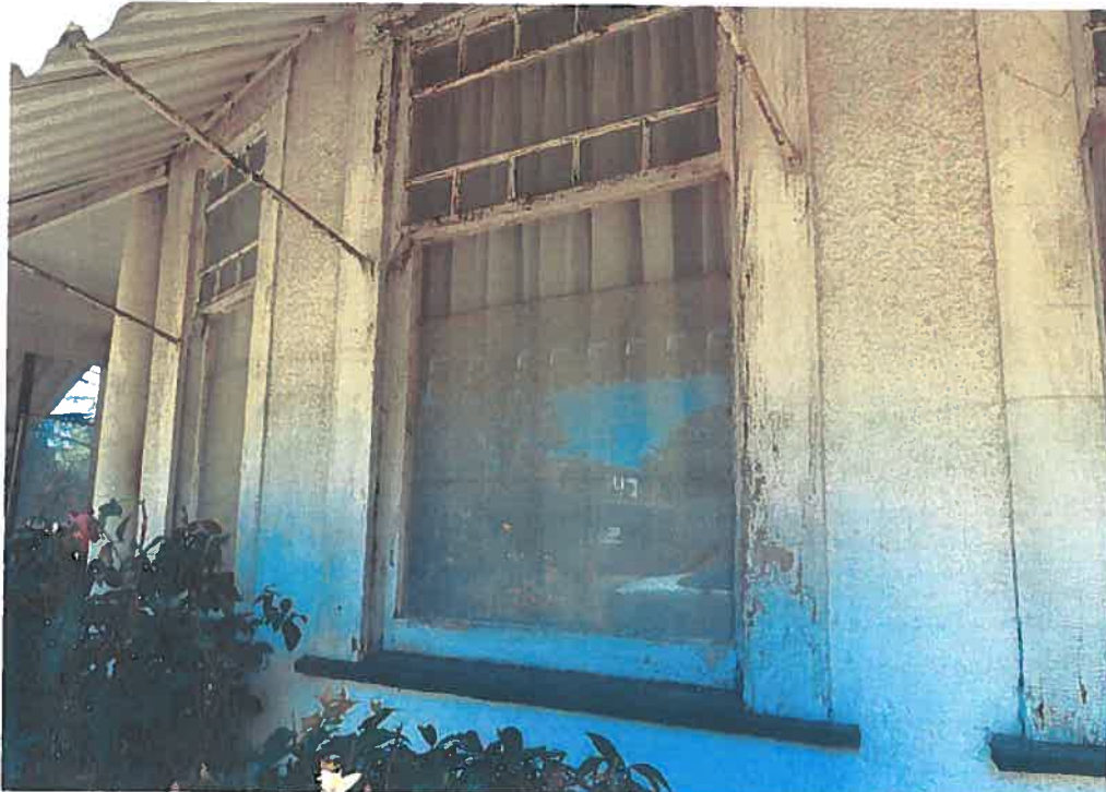
Detail of bay window at primary (south) façade, July 16, 2010 (Architectural Resources Group)
